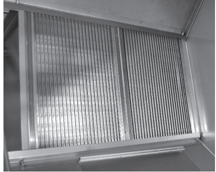
Plate recuperator (Fig. 12)
